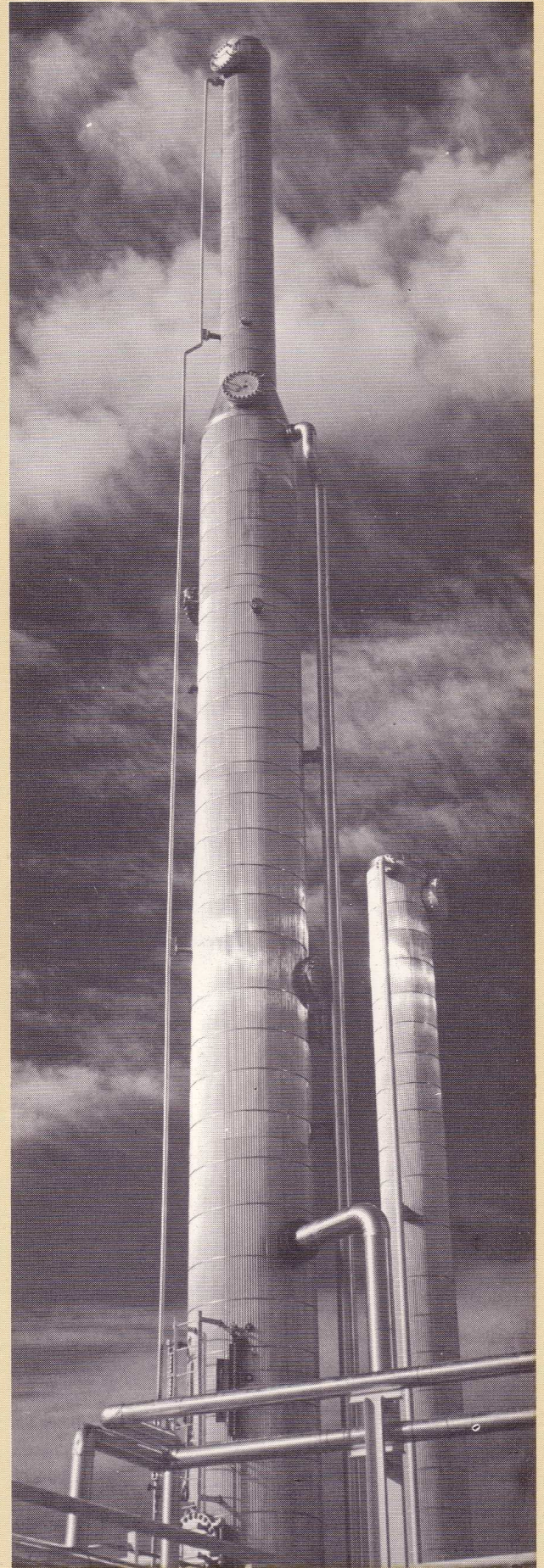
Rocket-like tubes belong to the Texas Gas and Oil Company's plant at Custer City, Oklahoma. Plant manufactures petroleum gas from natural gas.
